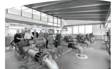
Nanaimo Reservoir No. 1 and Energy Recovery Facility – A Clean Energy Project Associated Engineering
