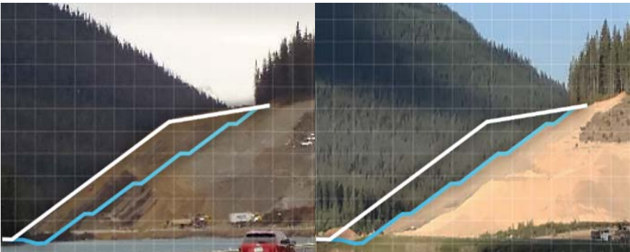
The massive 'Wapta Cut,' supplying over 500,000m 3 of material. GPS-equipped excavators were used to get precise cuts.
