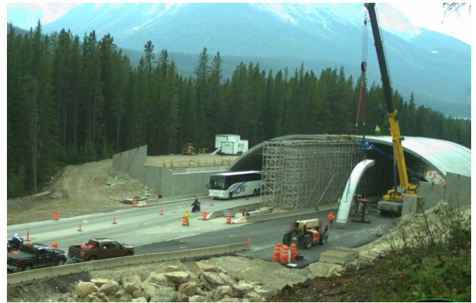
Construction of the 60m wide 34m span animal overpass, designed by COWI Bridge.
